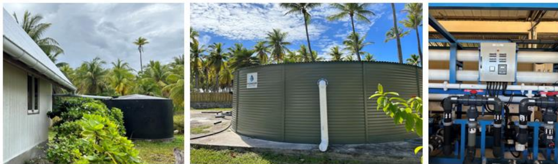
Figure 39. Water tanks and desalination facility in Rangiroa accommodations
