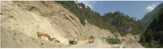
Construction is underway to build in lanes for the Kullu Highway. [Photo courtesy of Aditi Chanchani]
